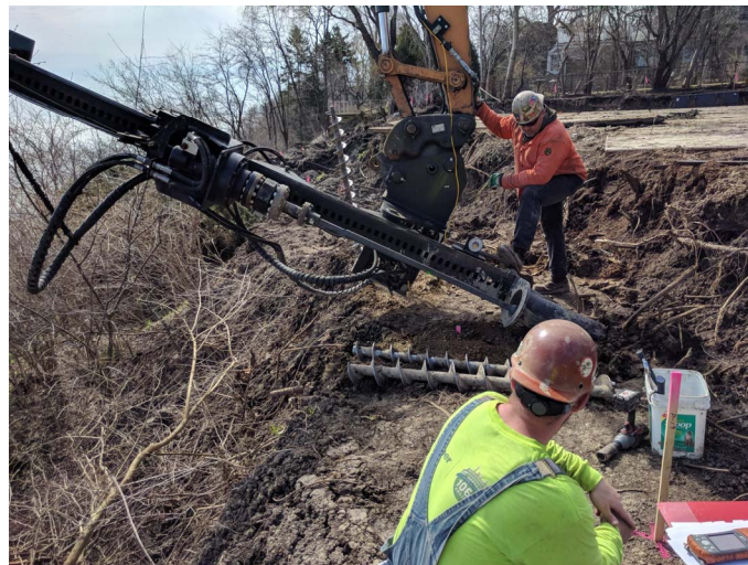
Fig. 2. Installation of screw piles (helical anchors) to be used as tiebacks in a slope stabilization project
